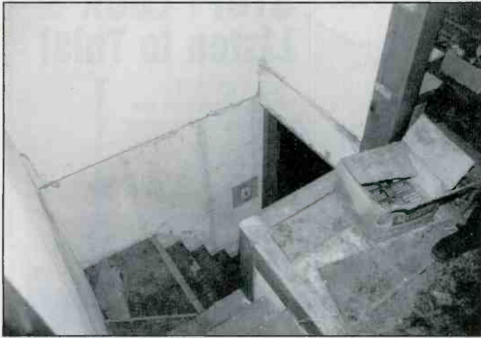
The radio shop was on the second floor, and was the center of activity in the old farmstead. These steep and rickety steps lead the way, and must have been a challenge for those carrying up larger console sets.
